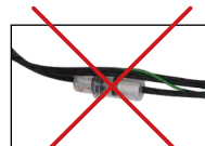
Water trap NOT OK
